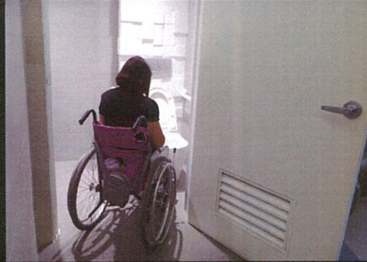
Wheelchair cannot enter due to obstruction and door cannot close
